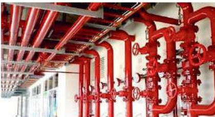
Fire Fighting System
