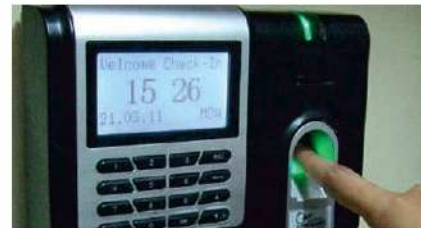
Biometric Access Control for lobby
