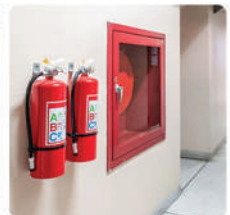
Fire Fighting System
