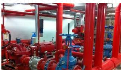
Fire Fighting System
