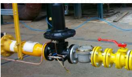
Centralized Gas Supply
