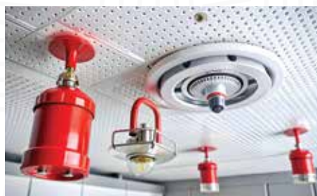
Fire Fighting System
