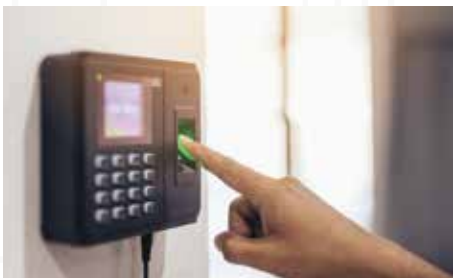
Biometric access Control for lobby
