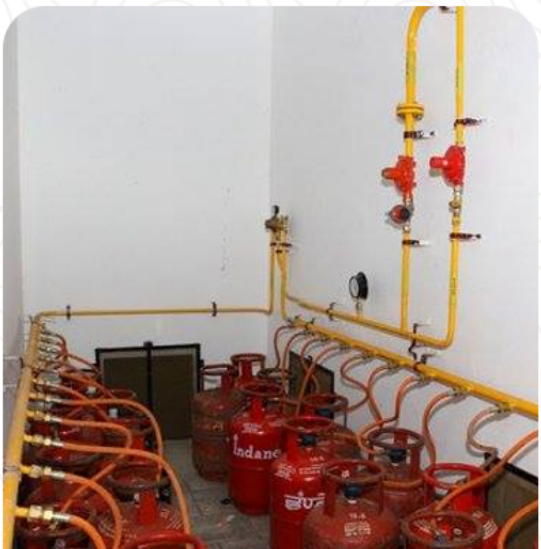
CENTRALIZED GAS SUPPLY
