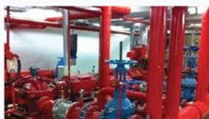
Fire Fighting System
