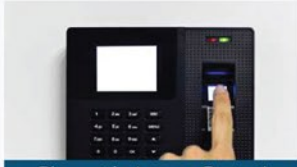
Biometric Access Control for lobby
