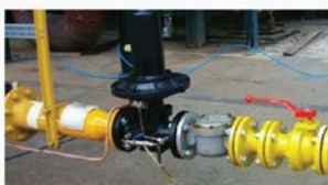
Centralized Gas Supply
